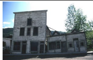
Figure 4 from tour: This damaged building in Dawson City, Canada, shows what can happen when the warm interior of a building causes the permafrost underneath to thaw. Credit: Andrew Slater.
